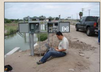
Azim start the process of programming the RTU and SCADA equipment
