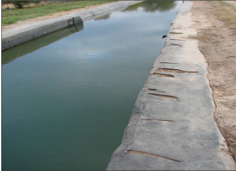
Figure 6. Cuts/tears in a rubber liner
