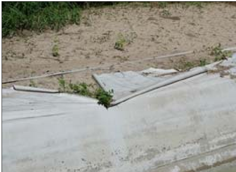
Figure 5. PVC Alloy liner damaged on the exposed area
