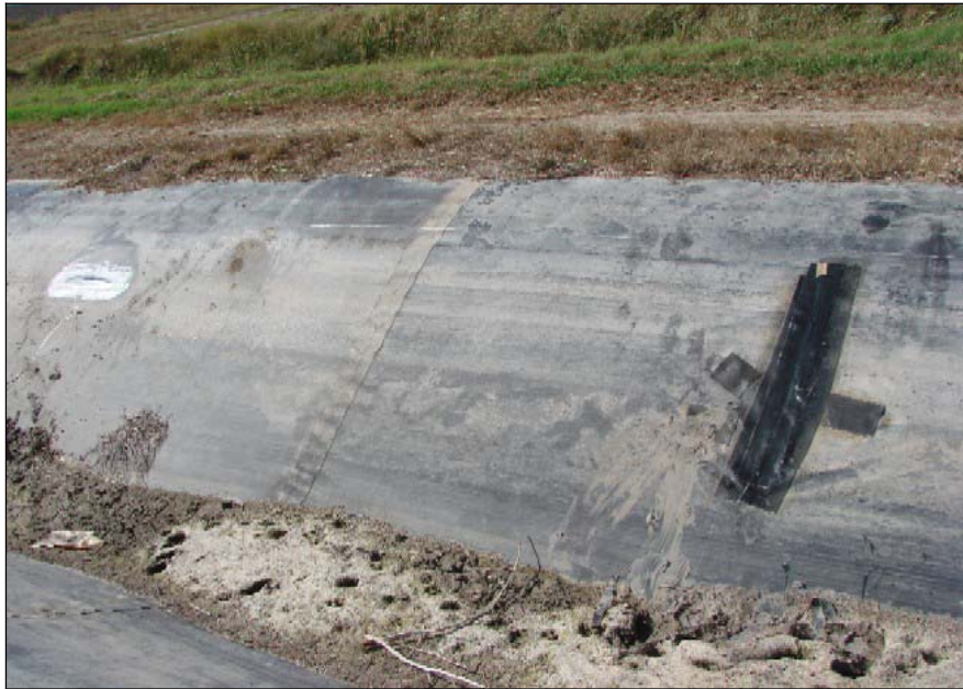
Figure 18. Sedimentation at the bottom of a lined canal
