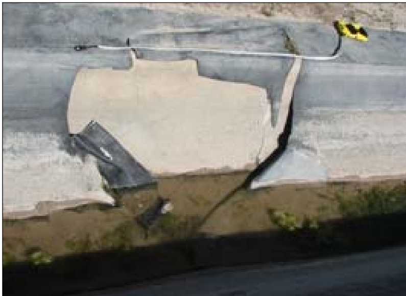
Figure 7. A rubber liner damaged possibly due to vandalism
