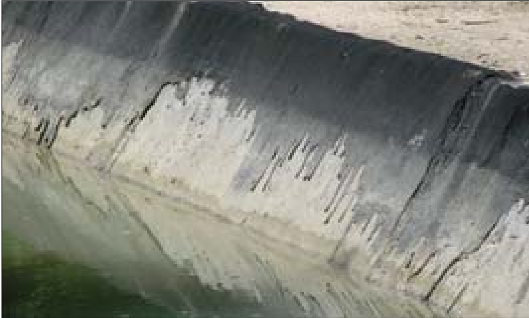
Figure 9. Residue left from a deteriorated polyurethane liner
