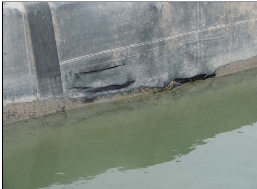
Figure 13. Horizontal cuts likely due to vandalism on the canal sidewall
