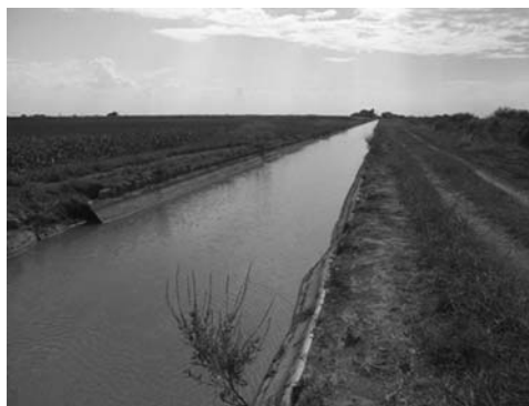
Figure 5. Ground-level photograph of a concrete canal section in the Delta Lake Irrigation District (Case 1)
