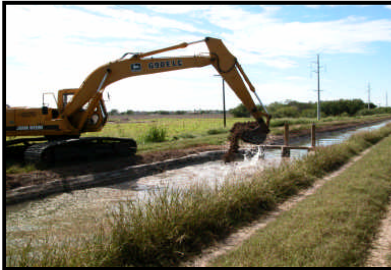
Figure A2. Typically, the irrigation district provides the equipment and constructs the earthen dams used to block off the ends of the test segment.
